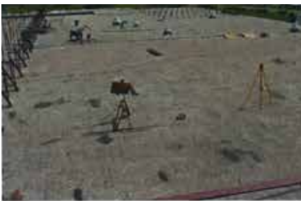
Existing ponding, leaking roof
